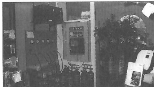
Automatic Blending Station at Facility of Holdive International, Amsterdam
